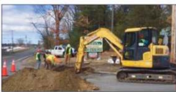
Baltzar Construction is seen doing working on the Feeding Hills Rd. project, right on the corner of Hudson Dr. (Photo by Greg Fitzpatrick)
